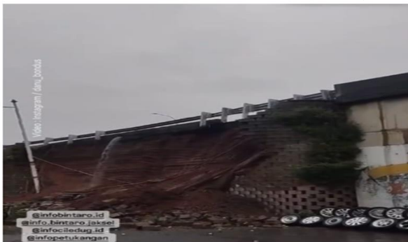
(e) Landslide on Sunday, July 7, 2024 Bintaro Toll Location.
