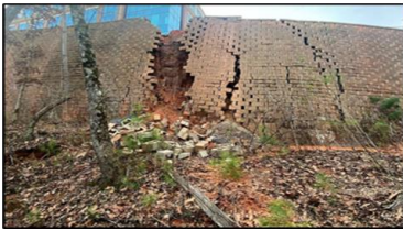
(c) Toe Failure MSE Wall due to hydrostatic pressure and long duration of rain
