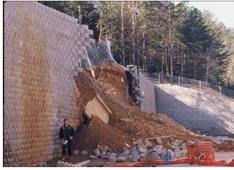
(a) MSE Wall collapsed due to hydrostatic pressure
