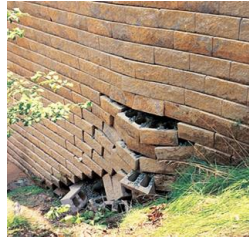
(b) Retaining wall collapse in Kelowna British Columbia, built in 2009, movement occurred on Nov 28, 2011
